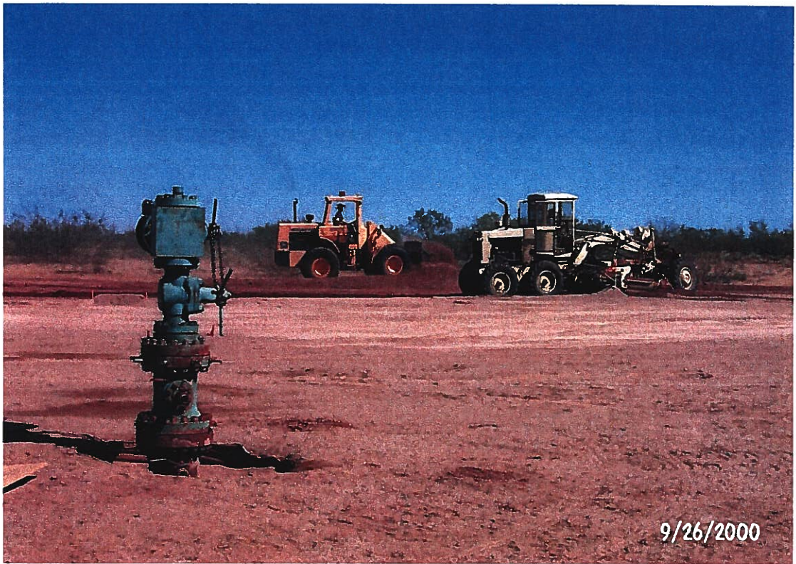
Photograph 32– Lake Meredith Salinity Control Project: RBM Incorporated is excavating the injection well facilities containment basin. The injection well Xmas Tree is in the foreground. Top of Xmas Tree has been rotated so the inlet now is to the east for future hookup to the injection pump discharge line. Photographed 9/26/2000 by Dennis McDonough.
