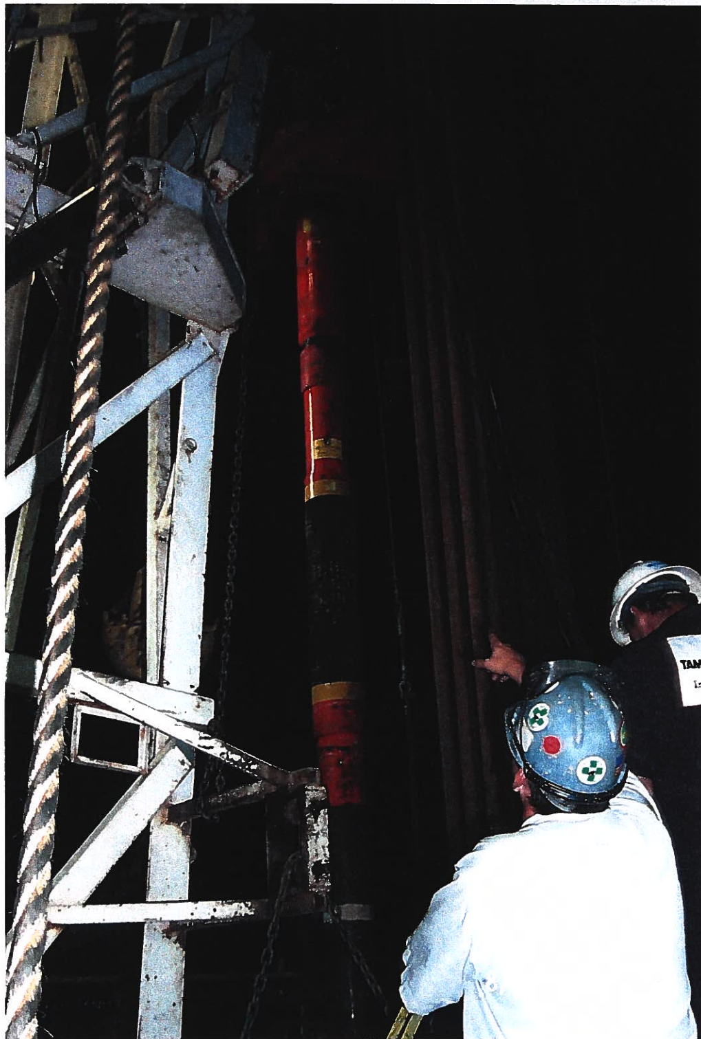
Photograph 15 – Lake Meredith Salinity Control Project: An external casing packer (ECP) and port collar are being lowered into the injection well. Photographed 8/1/1999 by Dennis McDonough
