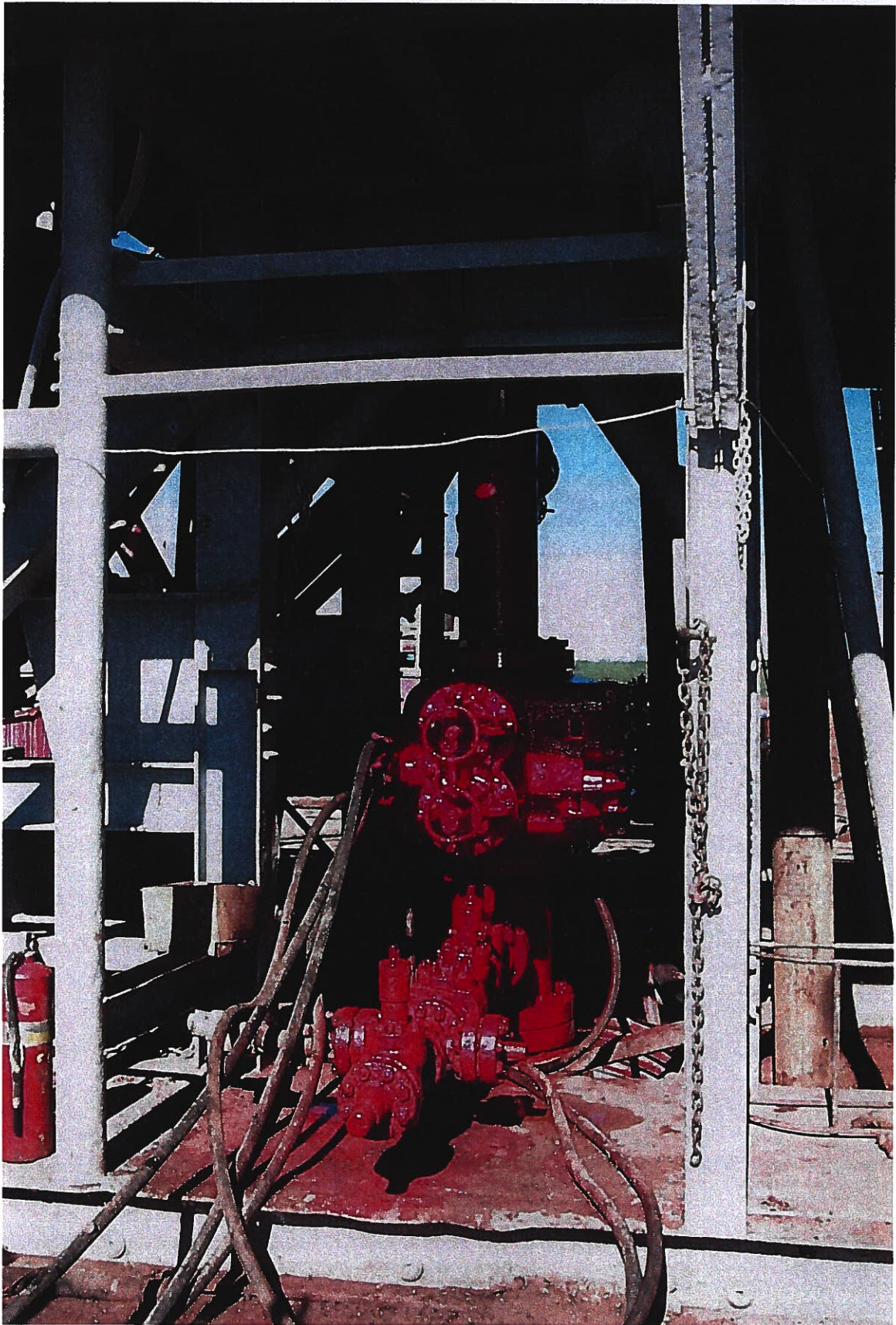
Photograph 8 – Lake Meredith Salinity Control Project: The blowout preventer has been installed on top of the Braden Head at Injection Well No. 1. Photographed 7/24/1999 by Dennis McDonough.
