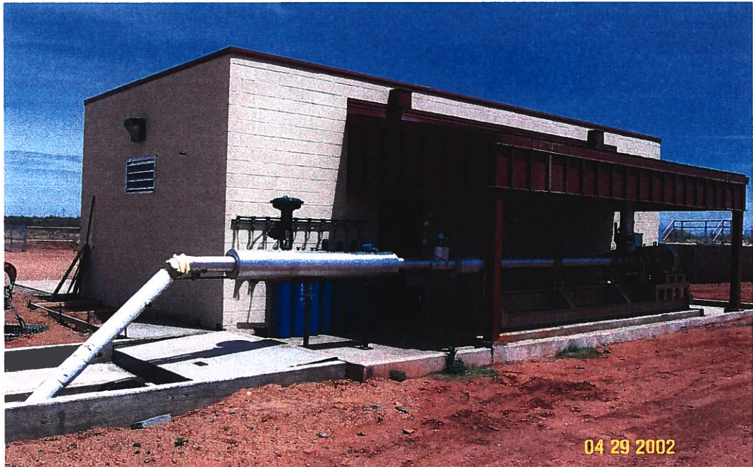
Photograph 49 – Lake Meredith Salinity Control Project – Filtered brine water is pumped to the injection well by the injection pump at the right. The discharge line from the pump travels along the concrete lined well chase. Photographed 4/29/2002 by Dennis McDonough.
