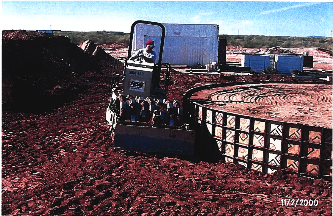
Photograph 38 – Lake Meredith Salinity Control Project: RBM Inc. employee is compacting backfill in the containment basin outside a brine water storage tank foundation wall. Photographed 11/2/2000 by Dennis McDonough.
