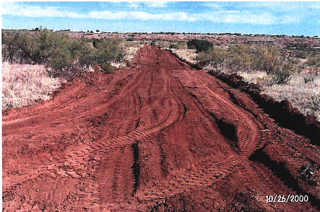
Photograph 22 – Lake Meredith Salinity Control Project: The Cat 950F loader in background is clearing the West Branch pipeline alignment prior to trenching operations. View is to north on land owned by Mr. Romero. Cleared width is about 18 feet. Photographed 10/26/2000 by Dennis McDonough.
