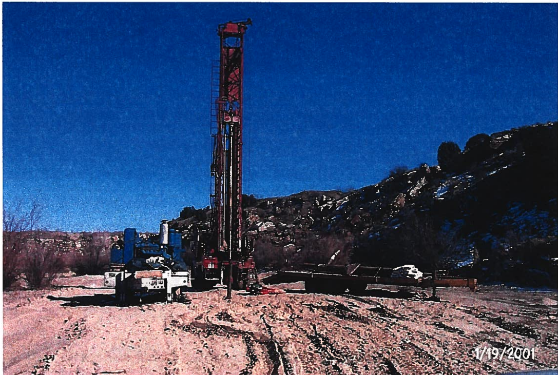
Photograph 20 – Lake Meredith Salinity Control Project: Hydro-Geologic set up their Star 30K drill rig at PW1-5. The Star 30K uses 4-1/2 inch drill pipe. A plastic membrane has been placed under the rig and the separate trailer-mounted triplex mud pump (blue pump on white trailer to left of rig). A 10-inch down-the-hole hammer stands vertically behind the rig. Photographed 1/19/2001 by Dennis McDonough.
