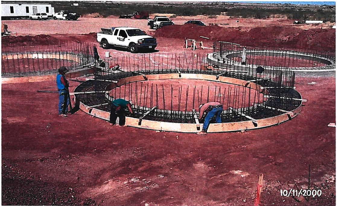
Photograph 33 – Lake Meredith Salinity Control Project: A Garney Companies, Inc. crew is installing rebar for a storage tank foundation in the injection well facilities containment basin. Photographed 10/11/2000 by Dennis McDonough.
