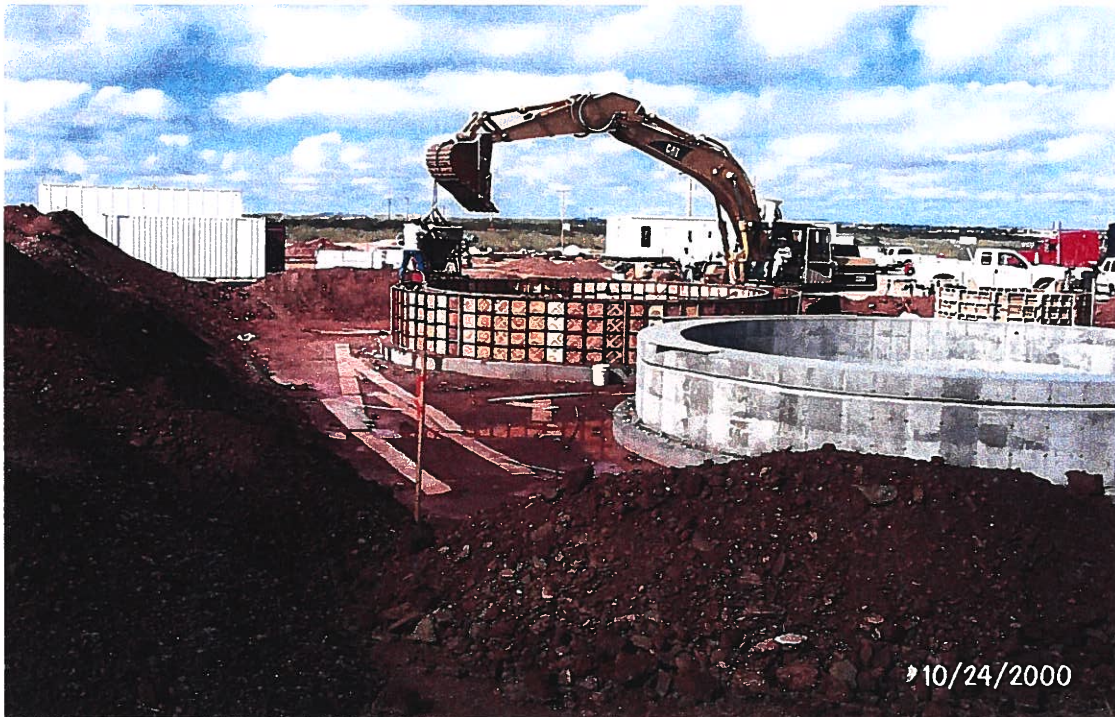
Photograph 35 – Lake Meredith Salinity Control Project: Concrete is being placed in a foundation wall for a brine water storage tank in the containment basin. Photographed 10/24/2000 by Dennis McDonough.
