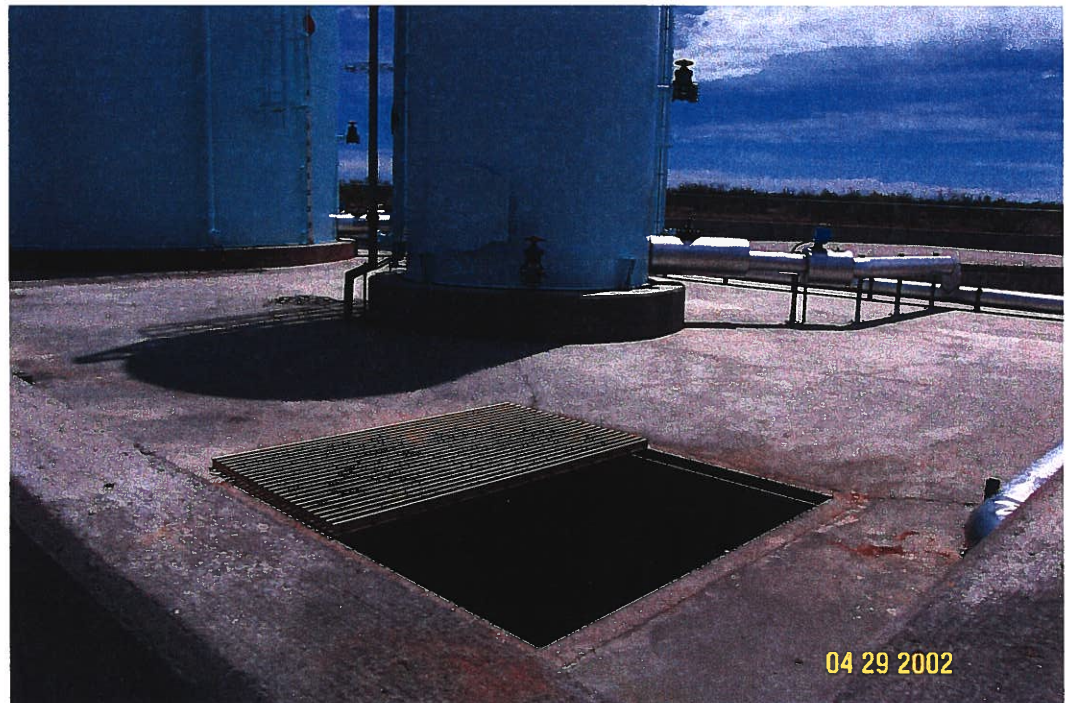
Photograph 45 - Lake Meredith Salinity Control Project: The containment basin sump is in the foreground with the 12,105-gallon run tank behind. A 96,400-gallon brine water storage tank is to the left. Photographed 4/29/2002 by Dennis McDonough.
