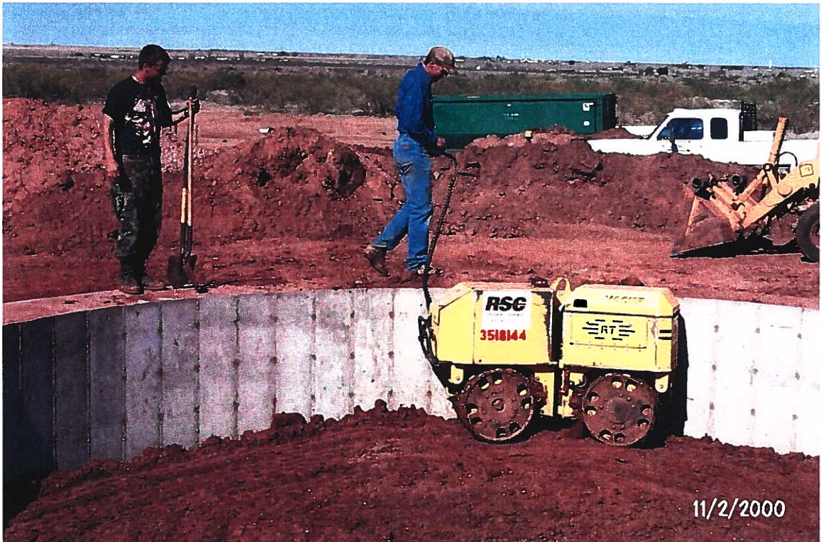
Photograph 37 – Lake Meredith Salinity Control Project: RBM Inc. operator is compacting backfill inside a foundation wall for a brine water storage tank. Photographed 11/2/2000 by Dennis McDonough.
