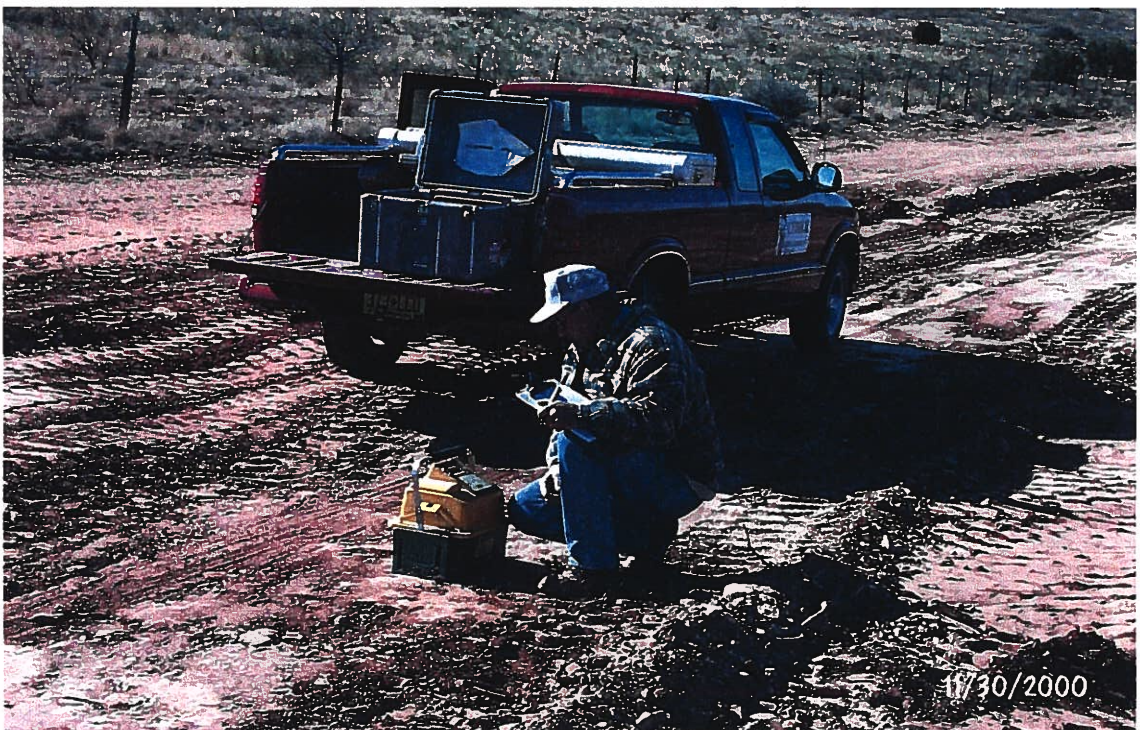
Photograph 26 – Lake Meredith Salinity Control Project: A Lydick Engineering & Surveyors technician is checking density of backfill material along the West Branch pipeline. Photographed 11/30/2000 by Jerry Osborn.
