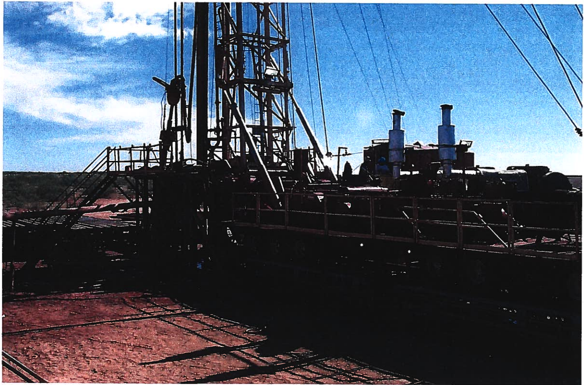
Photograph 2 – Lake Meredith Salinity Control Project: Drilling fluid return is processed in a series of tanks, shakers, and centrifuges (desilters) on the backside of the Norton drill rig at Injection Well No. 1. Photographed 7/23/1999 by Dennis McDonough.
