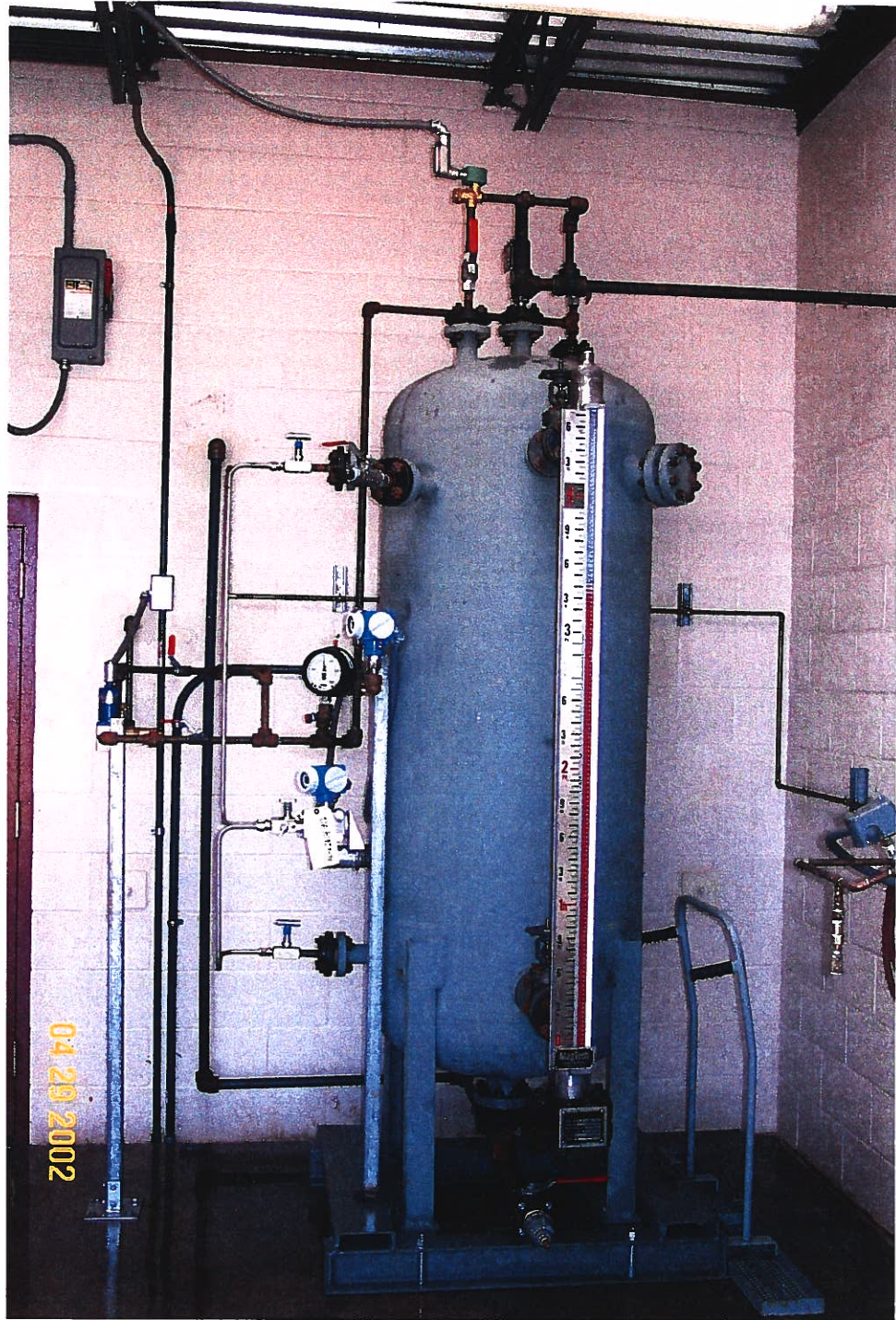
Photograph 51 – Lake Meredith Salinity Control Project: The seal pot is mounted in the corner of the injection building. It supplies pressurized fluid to the annular area of the injection well. The seal pot was subjected to rigorous testing before shipment by the manufacturer. The blue nitrogen tanks in Photograph 49 are used to pressurize the fluid. Photographed 4/29/2002 by Dennis McDonough.
