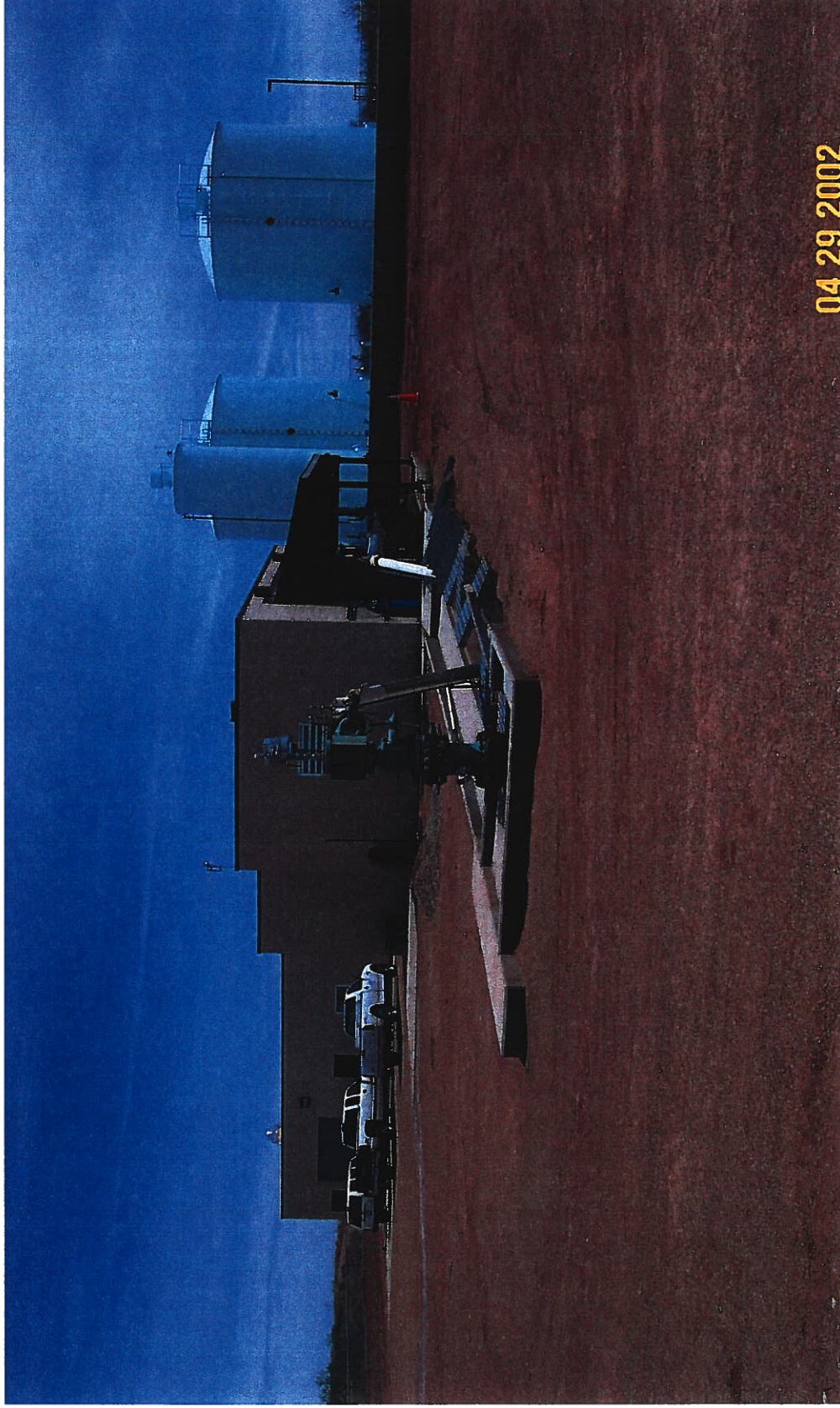
Lake Meredith Salinity Control Project – This view of the injection well facilities is to the northeast with injection well IW-1 in the middle foreground. The gratings have been removed from the discharge line (well chase) from the injection pump. CRMWA Corp. employees have added curbs to the well chase to prevent debris from entering. The injection pump and injection building are directly behind the injection well. The containment basin and storage tanks are to the right, and the office building is to the left. Photographed 4/29/02 by Dennis McDonough.
