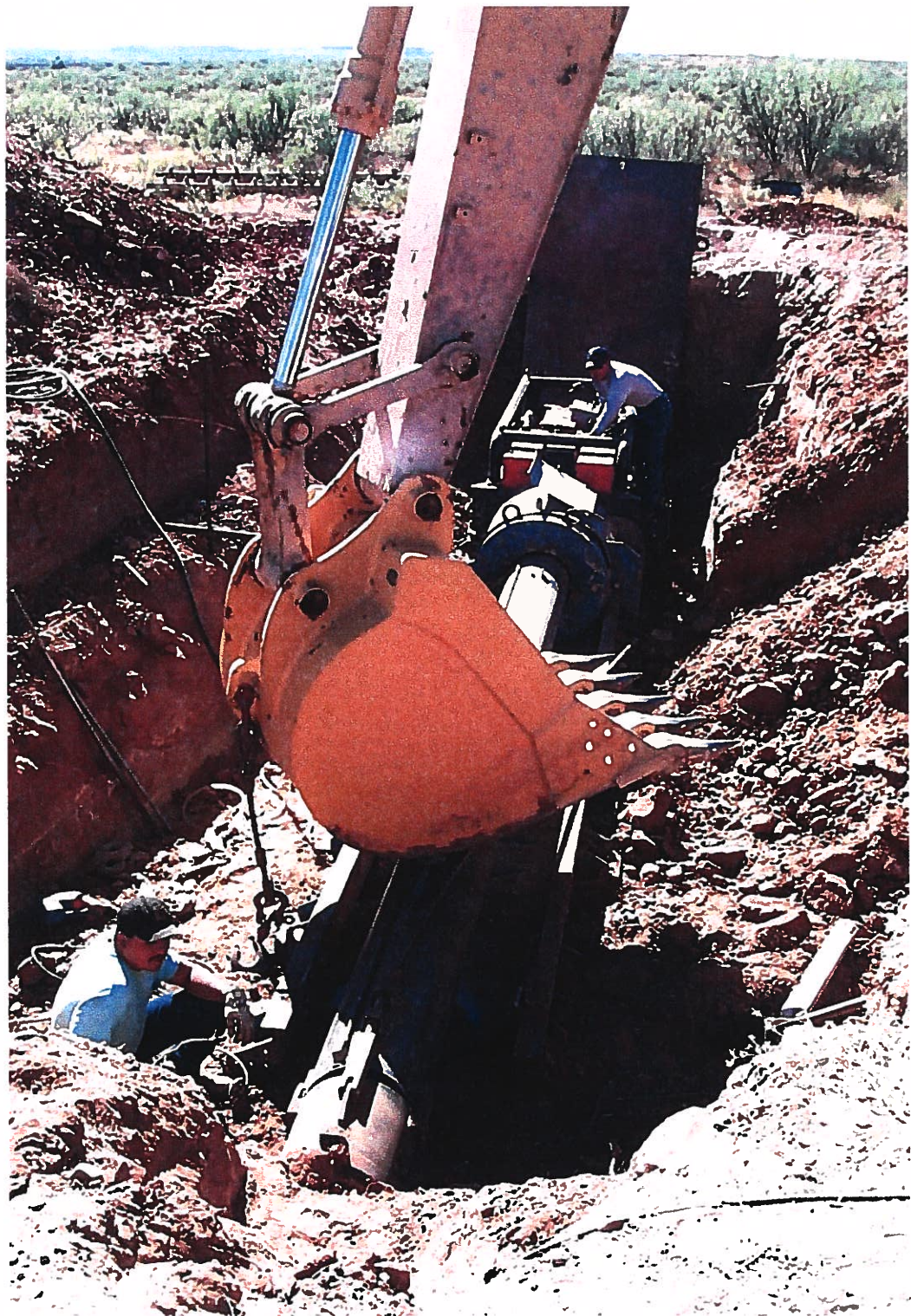
Photograph 31 – Lake Meredith Salinity Control Project: DH Underground, Inc. is starting the horizontal bore under Hwy 469. As casing is jacked, it is steered by pivoting the section in foreground. A cutting head and auger system remove cuttings. Extra flight augers are at top of picture. The top of casing is only a few inches below a fiber optic cable. Photographed 10/11/2000 by Dennis McDonough.
