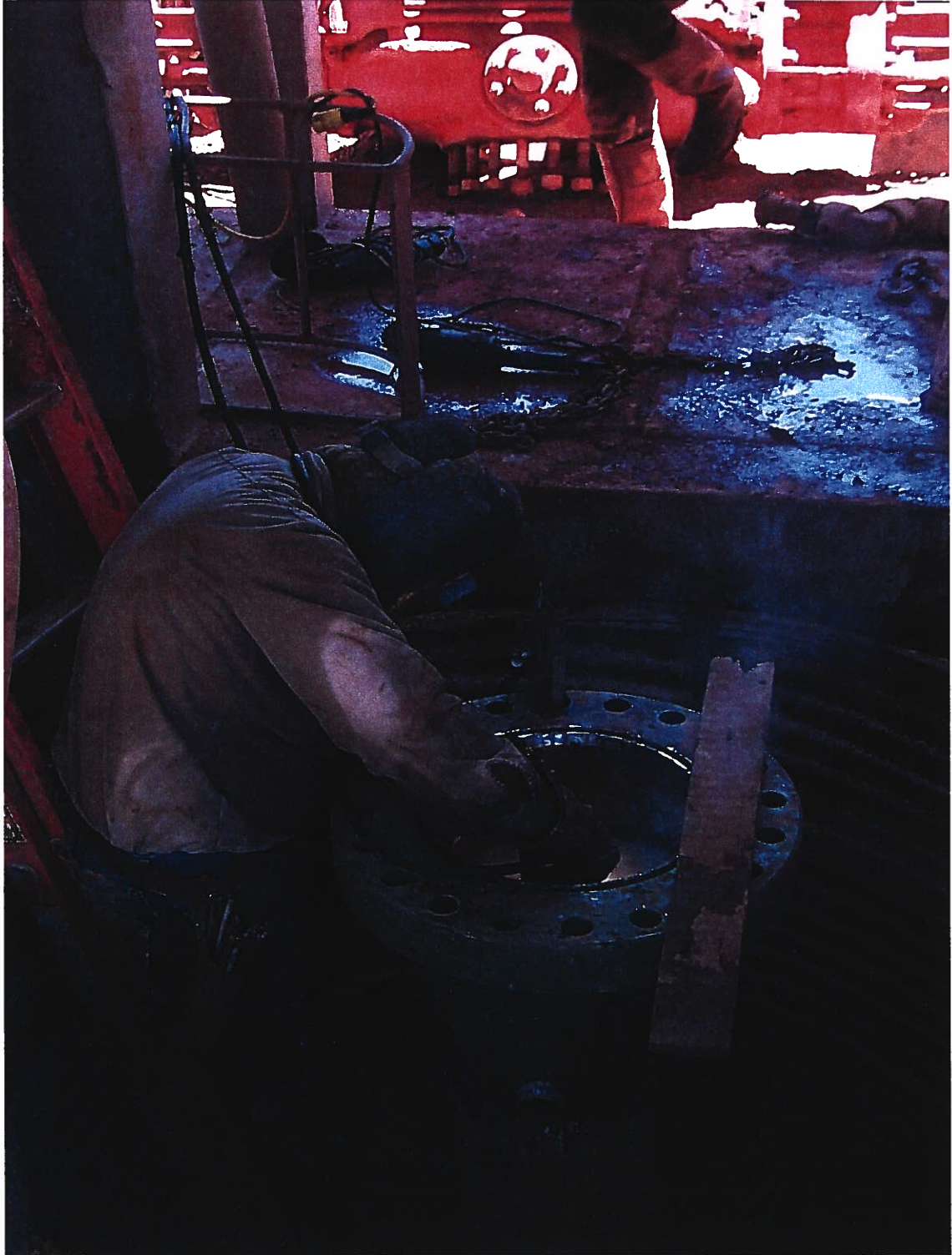
Photograph 6 – Lake Meredith Salinity Control Project: Welder is installing a Braden Head on 13-3/8" surface casing at Injection Well No. 1. The twenty-inch steel conductor casing has been cut off several feet below the Braden Head. Photographed 7/24/1999 by Dennis McDonough.
