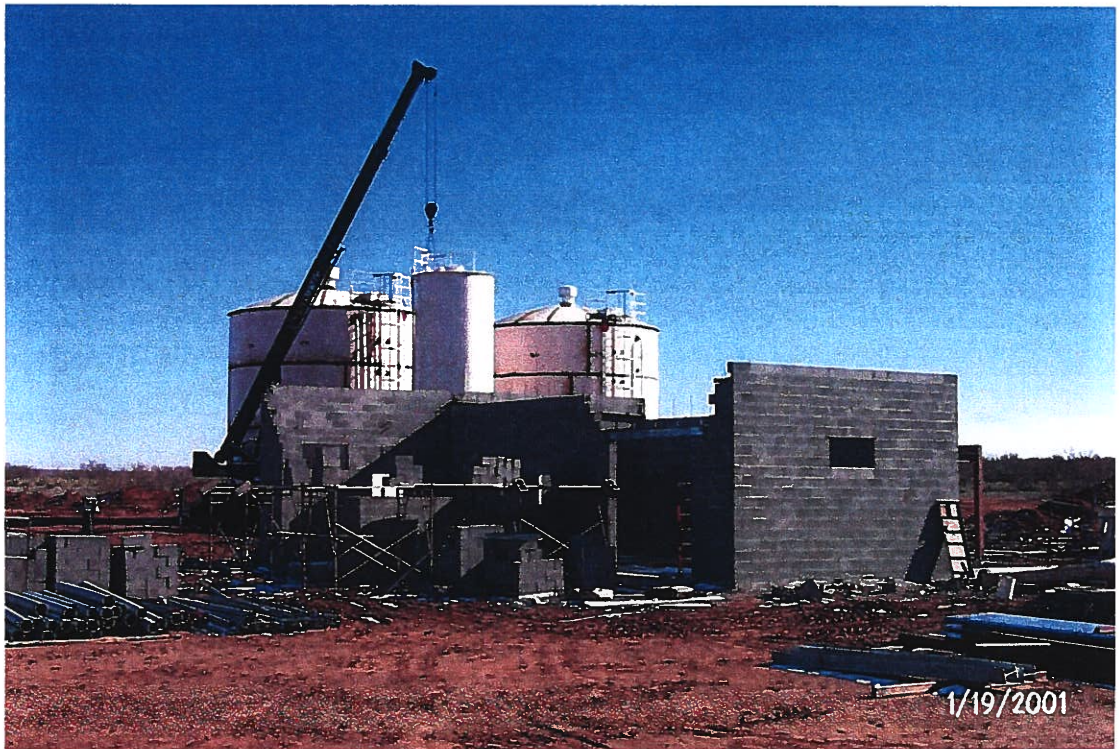
Photograph 39 – Lake Meredith Salinity Control Project: The 12,405 gallon “Run Tank” is being placed in the containment basin. The two 96,400 gallon brine storage tanks are to the right and left of the run tank. Erection of the masonry walls for the office building (left) and injection building (right) has been stopped due to cold temperatures. Photographed 1/19/2001 by Dennis McDonough.
