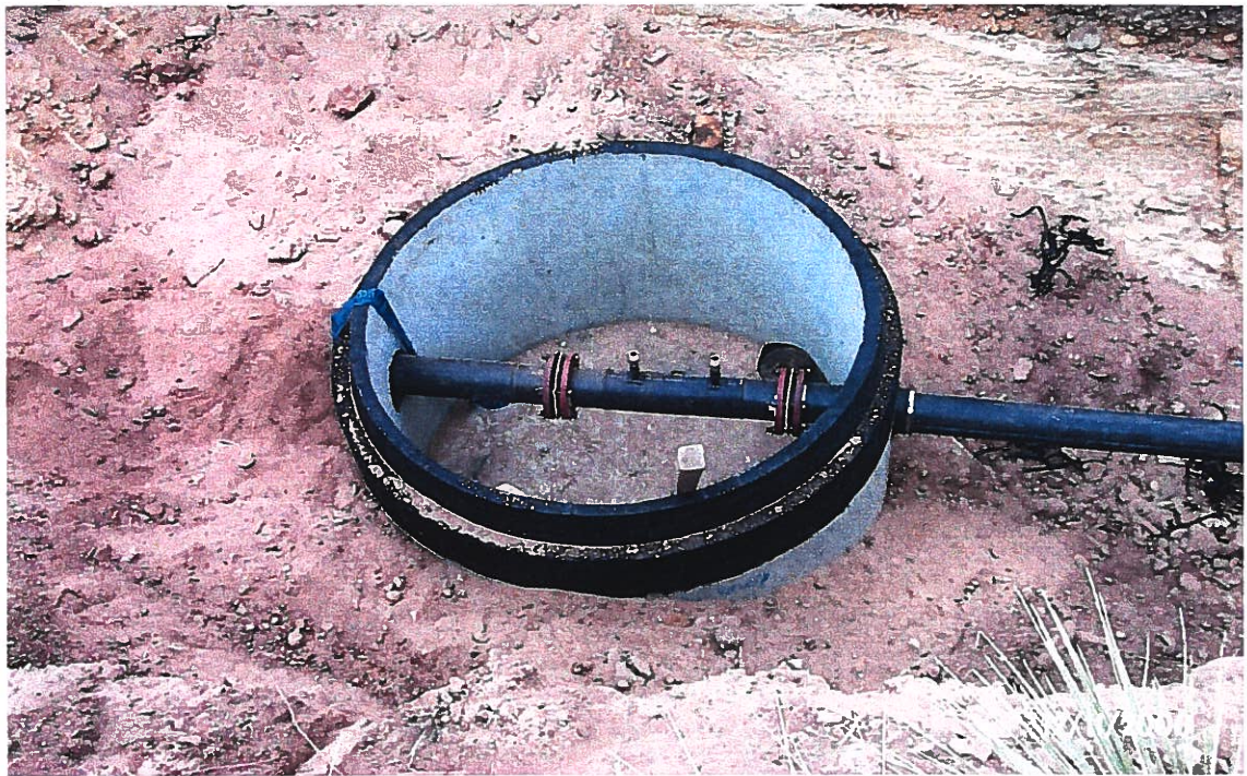
Photograph 27 – Lake Meredith Salinity Control Project: This valve vault is at Station 232+42.75 on the West Branch Pipeline. The vault is located at the top of plateau just before the pipeline drops off into the Canadian River valley floor. Photographed 12/11/2000 by Dennis McDonough.
