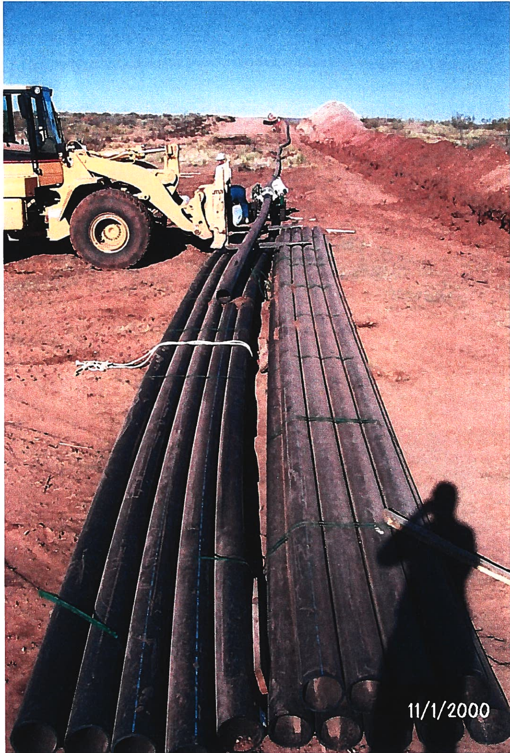
Photograph 24 – Lake Meredith Salinity Control Project: HDPE pipe sections are being welded near the containment basin. The trackhoe at the north end of the welded pipe is used to drag welded pipeline towards Hwy. 469. Photographed 11/1/2000 by Dennis McDonough.
