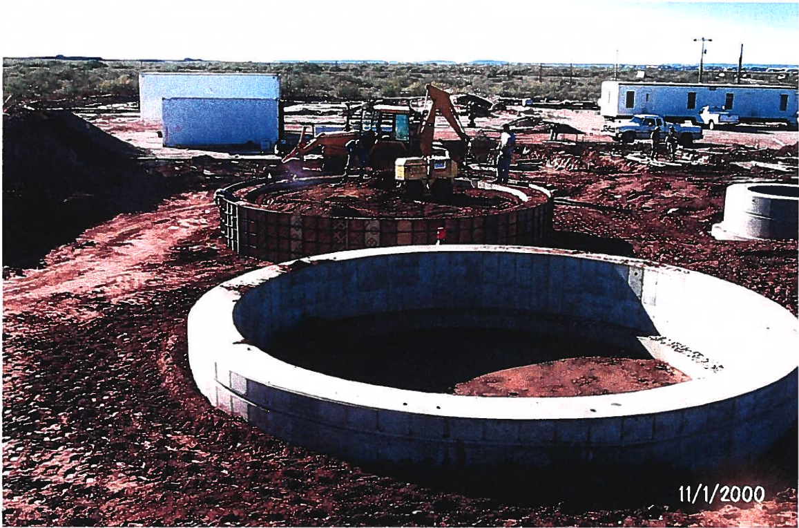
Photograph 36 - Lake Meredith Salinity Control Project: A remote-controlled compactor is being used to compact backfill inside the foundation of the future (no tank will be erected during Phase 2) tank foundation. A contract modification was to place a concrete cap over this backfilled foundation. Photographed 11/1/2000 by Dennis McDonough.
