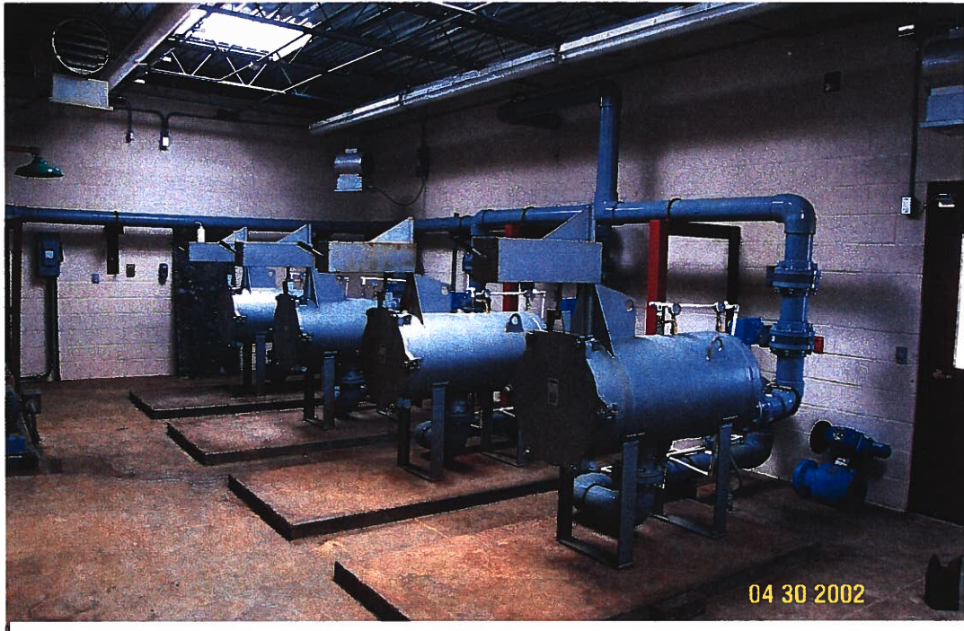
Photograph 48 – Lake Meredith Salinity Control Project – Brine water from the transfer pump is processed through this bank of cartridge filters. Photographed 4/30/2002 by Dennis McDonough.
