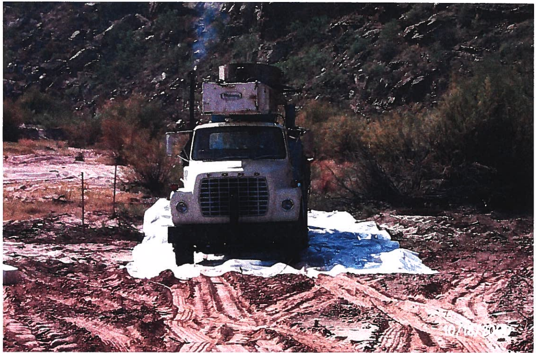
Photograph 19 – Lake Meredith Salinity Control Project: Couch Pump Service is backing their Midway 1300 drill rig onto a waterproof membrane at the site of PW1-1. Membranes and metal drip pans were used to prevent soil and water contamination from spills of fuel, oil, grease, or other chemicals. Photographed 10/19/2000 by Dennis McDonough.
