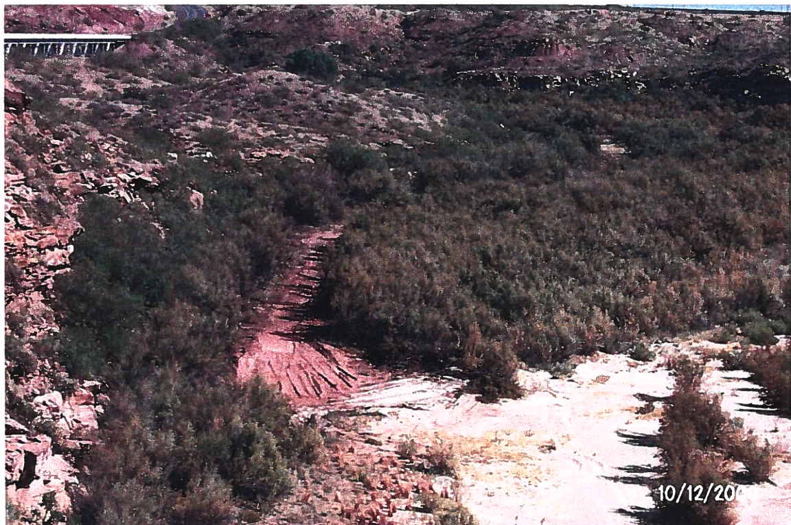
Photograph 18 – Lake Meredith Salinity Control Project – Couch Pump Service had a local subcontractor, Versatile Construction, clear a path through the salt cedars for access to production well PW1-1. This well is located below where trail ends just left of the lower center of the photograph. The Highway 54 bridge over the Canadian River is in the upper left corner of the photograph. Photographed 10/12/2000 by Dennis McDonough.
