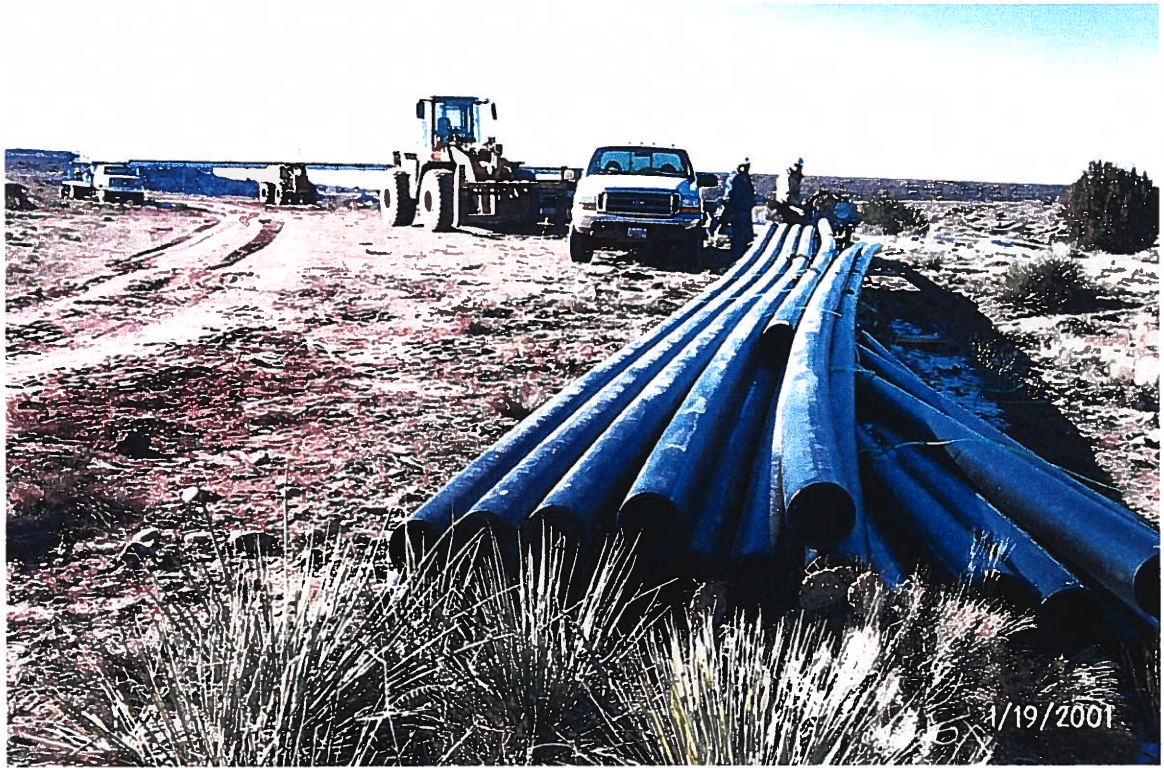
Photograph 30 – Lake Meredith Salinity Control Project: The Garney pipeline crew is welding 6-inch HDPE pipe for the East Branch Pipeline. View is to the west with the Union Pacific Railroad bridge over the Canadian River in the background. Photographed 1/19/2001 by Dennis McDonough.
