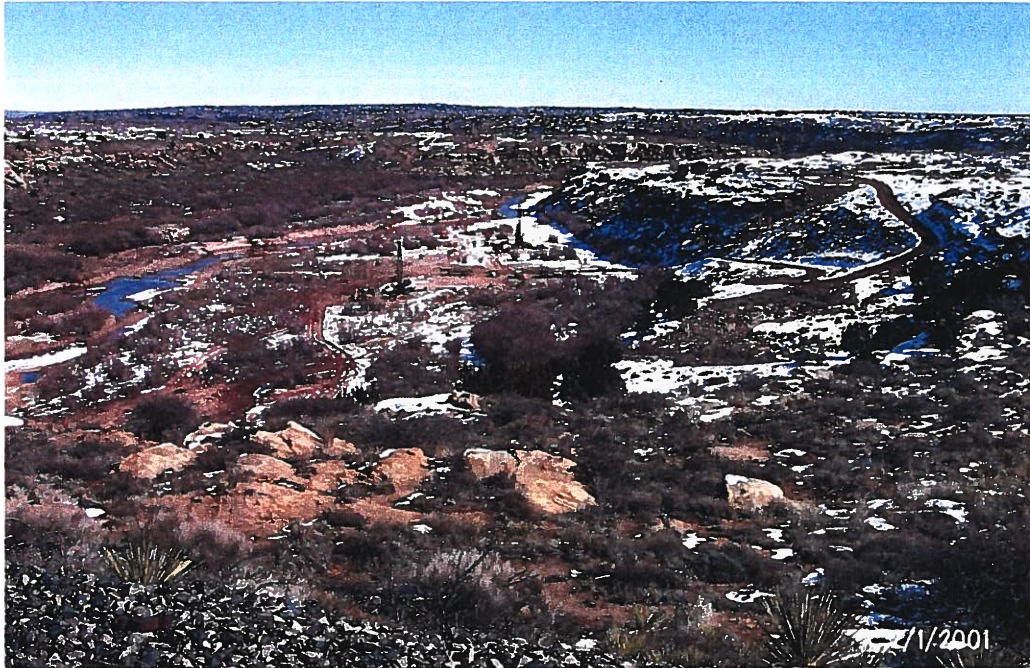
Photograph 21 – Lake Meredith Salinity Control Project: The Midway 1300 (closest to camera) and Star 30K drill rigs are set up on production wells PW1-4 and PW1-5 in the Canadian River valley. The view is to the east from the south abutment of the Union Pacific Railroad bridge. Photographed 2/1/2001 by Dennis McDonough.
