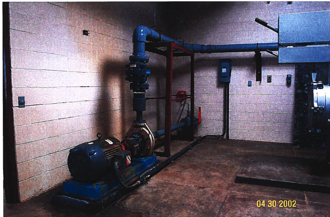
Photograph 47 – Lake Meredith Salinity Control Project: Brine water is piped from the storage tanks to the transfer pump and then to the cartridge filters to the right. Photographed 4/30/2002 by Dennis McDonough.
