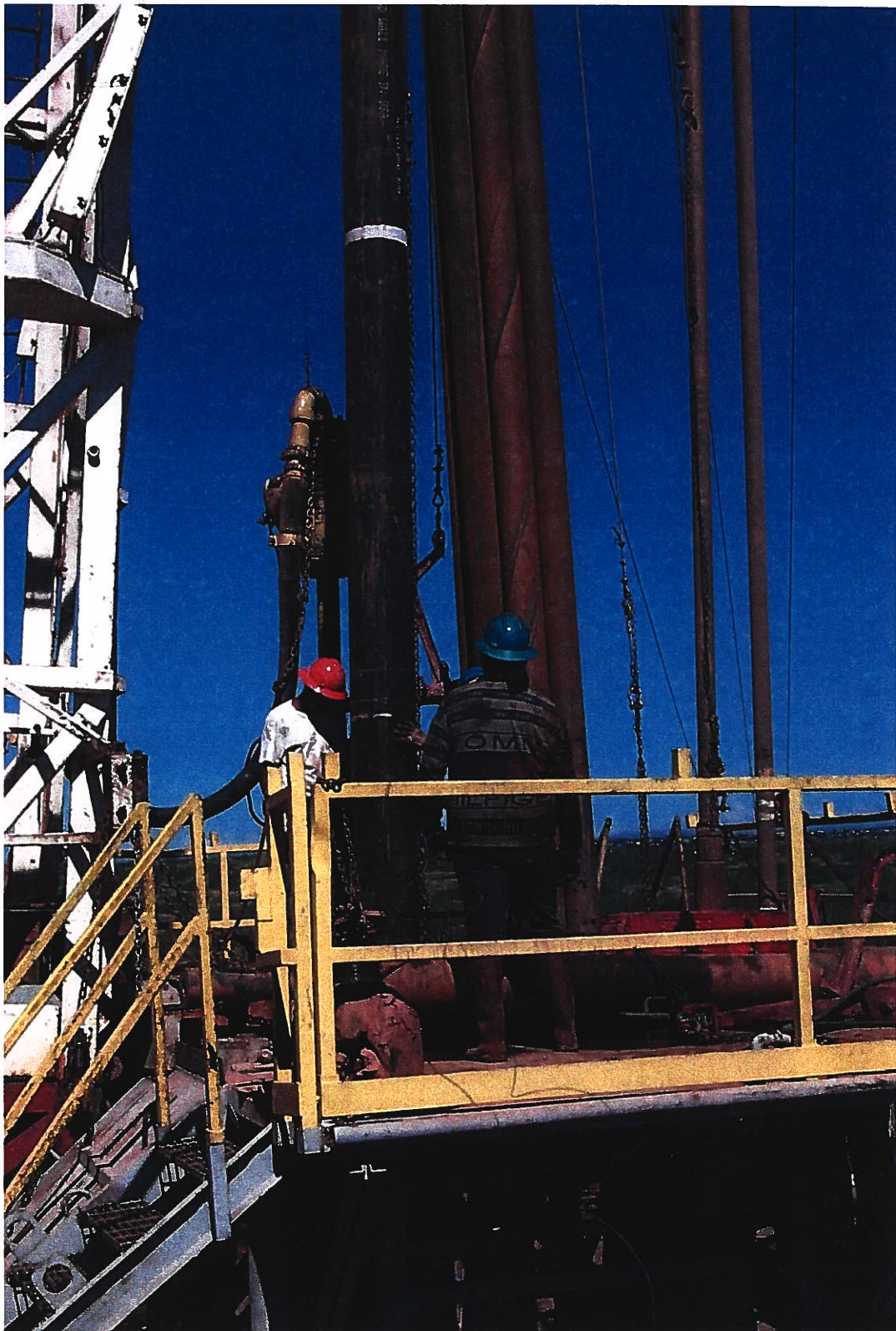
Photograph 5 – Lake Meredith Salinity Control Project: The drill crew is removing excess 13-3/8” surface casing after cement has set 24 hours at Injection Well No. 1. Photographed 7/24/1999 by Dennis McDonough.
