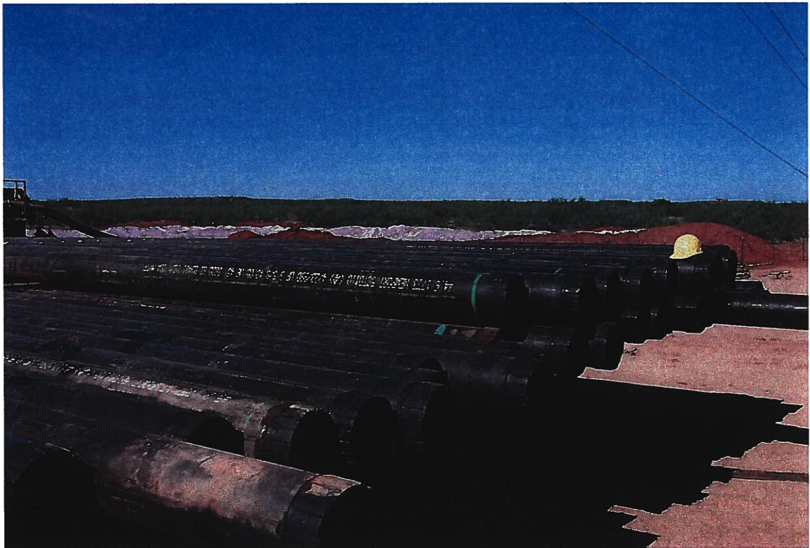
Photograph 4 - Lake Meredith Salinity Control Project: Steel protection (intermediate) casing, 9-5/8" O.D., has been tallied prior to installation at Injection Well No. 1. Photographed 7/23/1999 by Dennis McDonough.
