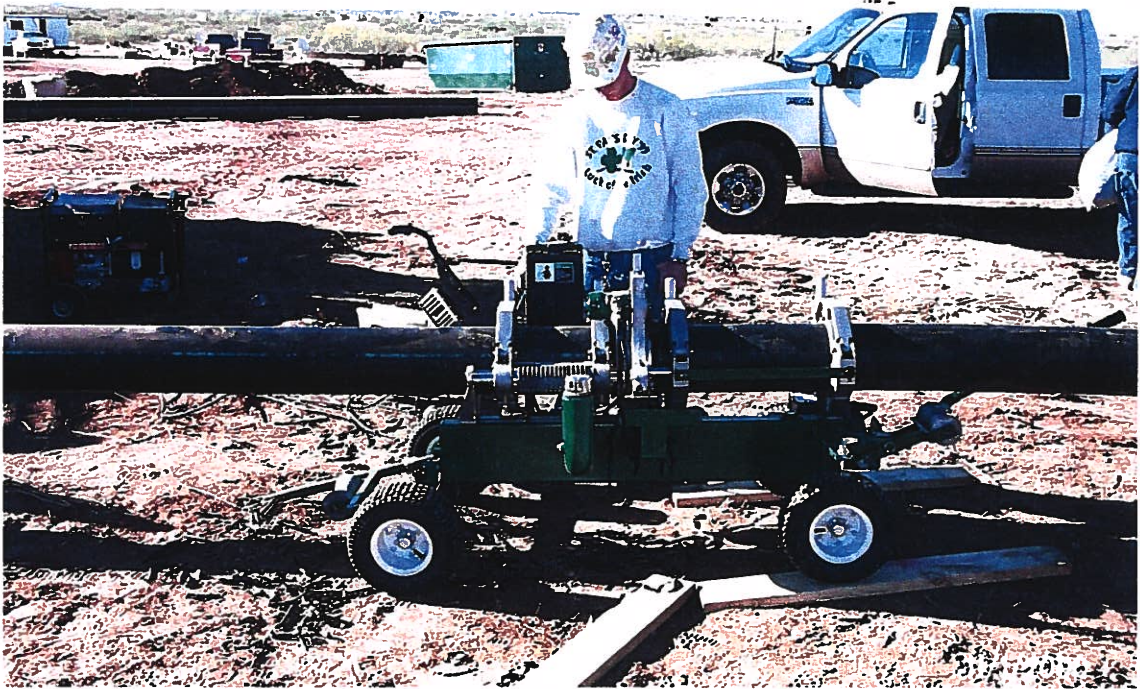
Photograph 25 – Lake Meredith Salinity Control Project: A Garney employee is trimming and welding 8-inch diameter HDPE pipe. Photographed 11/1/2000 by Dennis McDonough.
